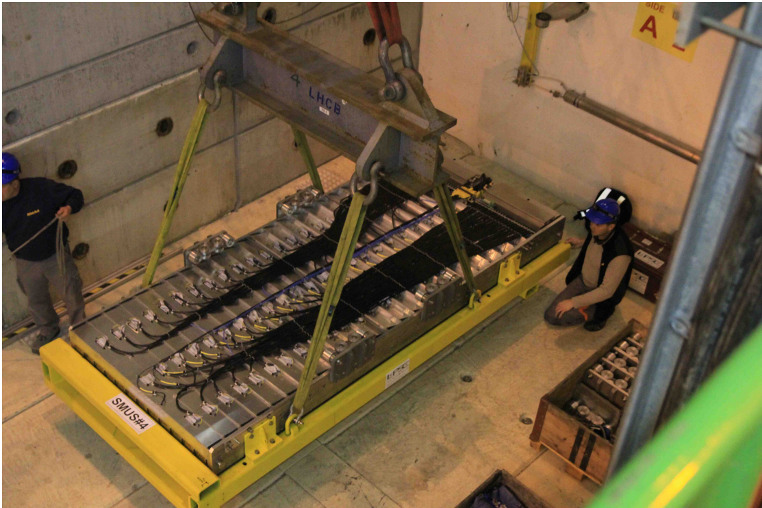
Fig. 2: View of one EMCal super-module during the installation into the ALICE detector. The cradle holds the 24 strip modules into a mechanically rigid unit. Each strip module holds 12 unit modules. On the right side the two electronics crates are visible.
